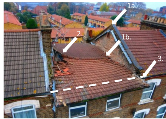
Fig. 1. The collapse of a roof in Tottenham, U.K., 2014. Picture from http://www.tottenhamjournal.co.uk/news/lunchbreak_saves_lives_of_builders_in_tottenham_roof_collapse_1_3858222 .
